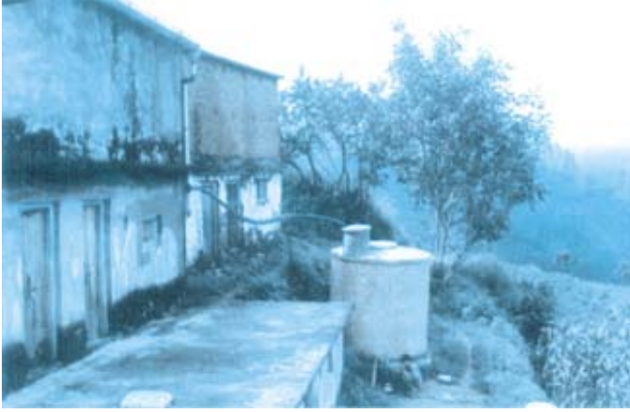
The rooftop rainwater can be fed into a tank through a pipe for meeting domestic needs
